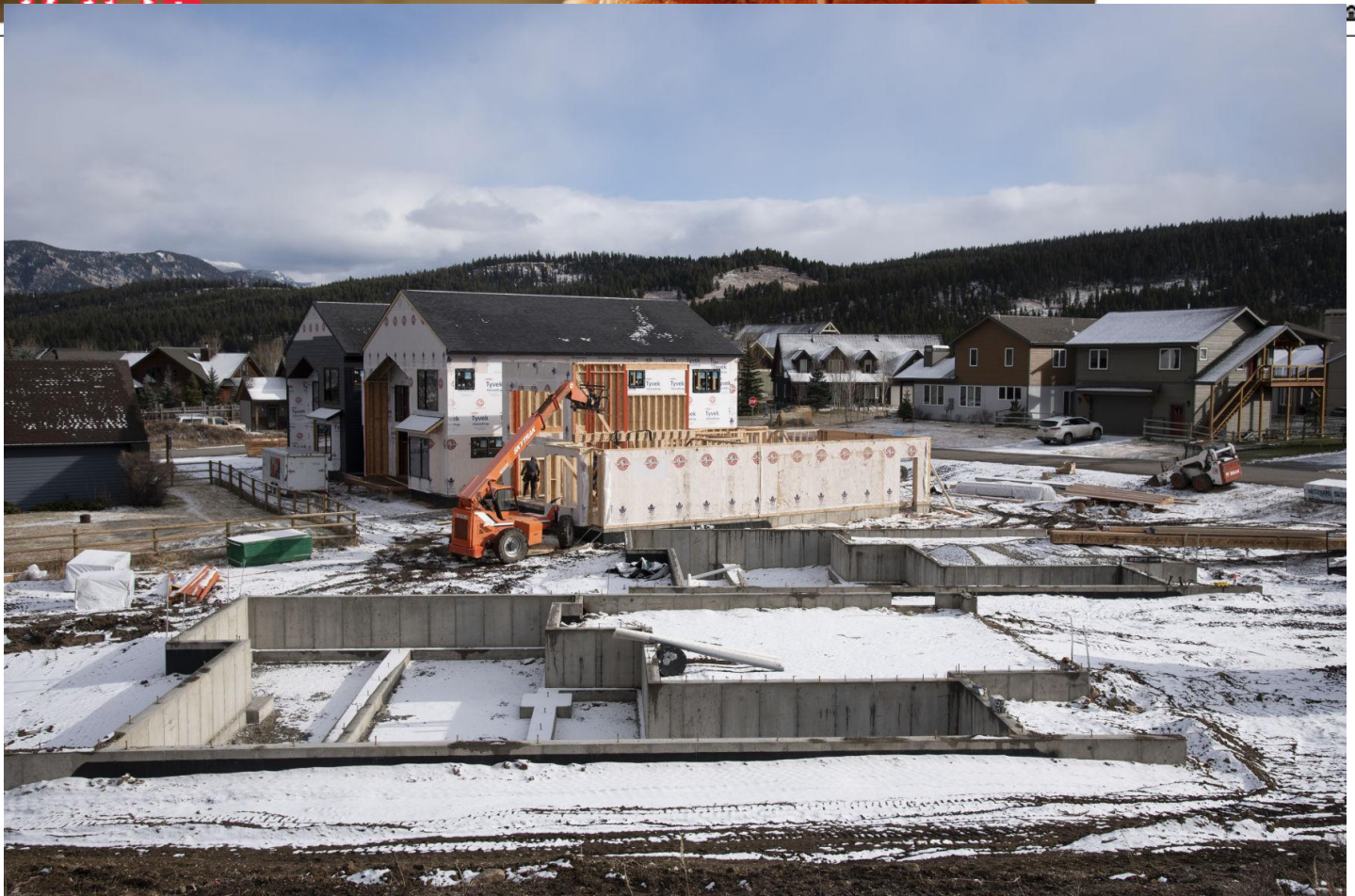
A row of houses in Big Sky in various stages of construction are dusted with snow on Wednesday, Nov. 10, 2021.
